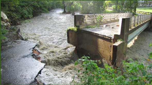
Damage to a road in Colrain during Tropical Storm Irene.
